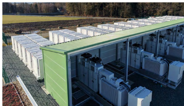
BESS Wunsiedel: operational since second half of 2025
