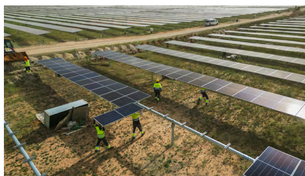
Operational since 2024: the Picón PV facility
