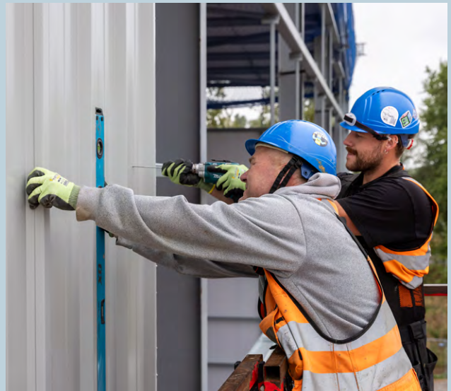
Installation of the façade cladding at the plastics recycling plant in Ellesmere Port
