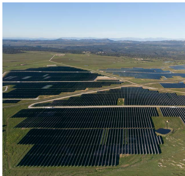
Operational since December 2023: the Trujillo PV facility (Cáceres region)
